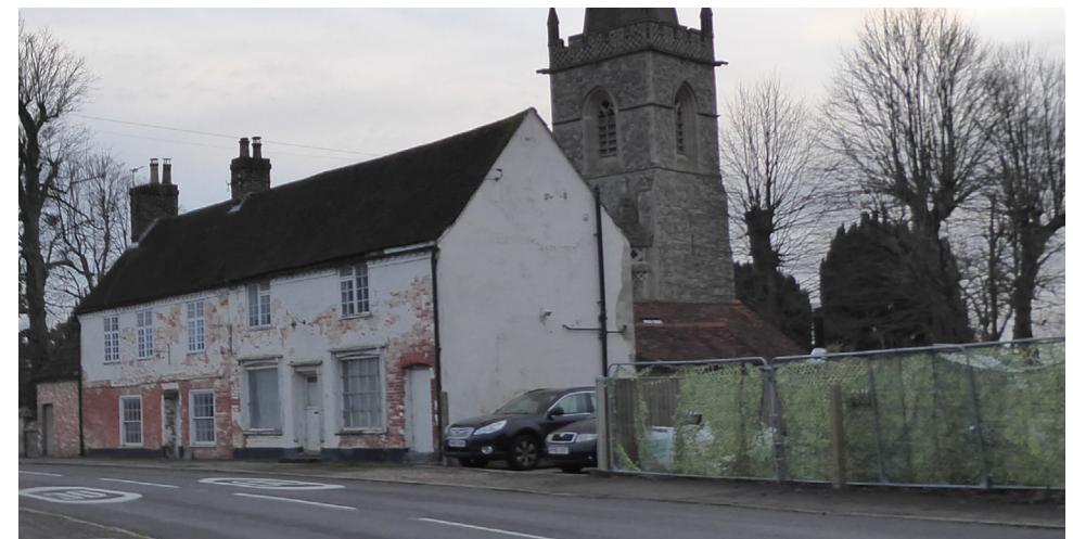
Figure 43 Church Cottage in state of disrepair and Heras fences at the boundary of Crown House
