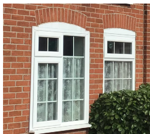
Figure 40 Loss of original features with the replacement of timber sashes and casement with uPVC
